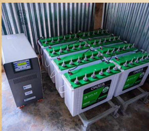
Solar inverter and batteries
