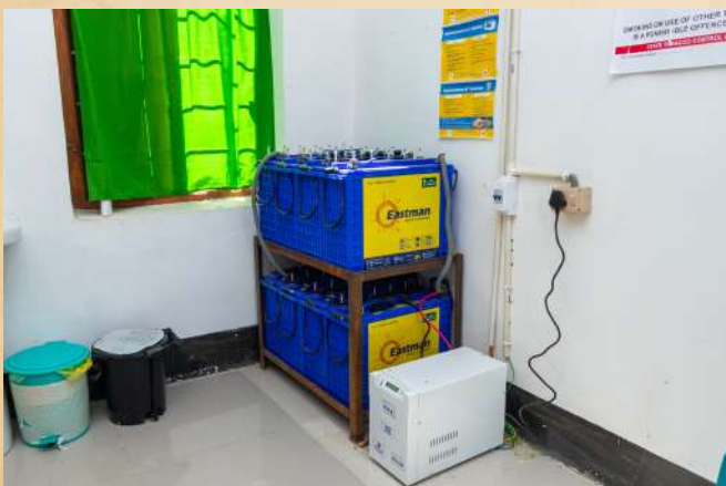
Solar inverter and batteries
