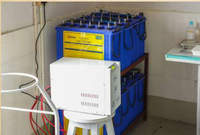
Solar inverter and batteries
