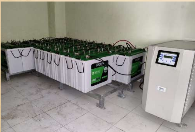
Solar inverter and batteries
