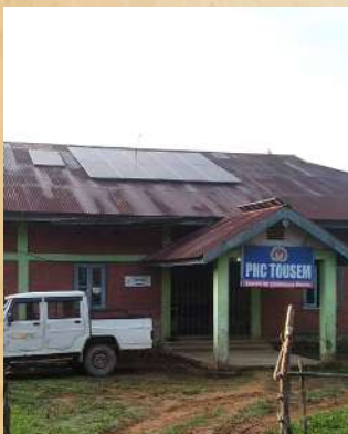
Solar Panel at PHC Tousem
