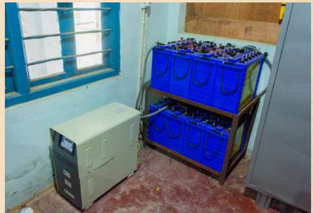
Solar inverter and batteries
