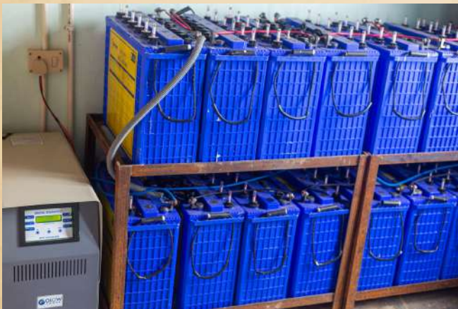
Solar inverter and batteries
