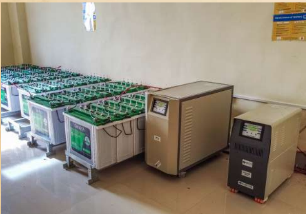
Solar inverter and batteries
