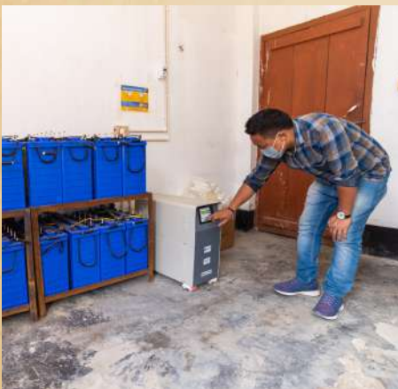
Solar inverter and batteries
