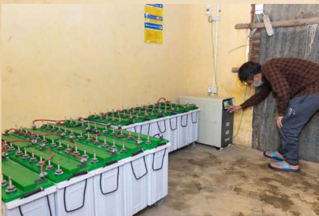
Solar inverter and batteries
