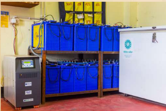
Solar inverter and batteries
