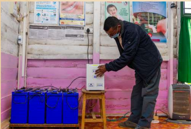
Solar inverter and batteries
