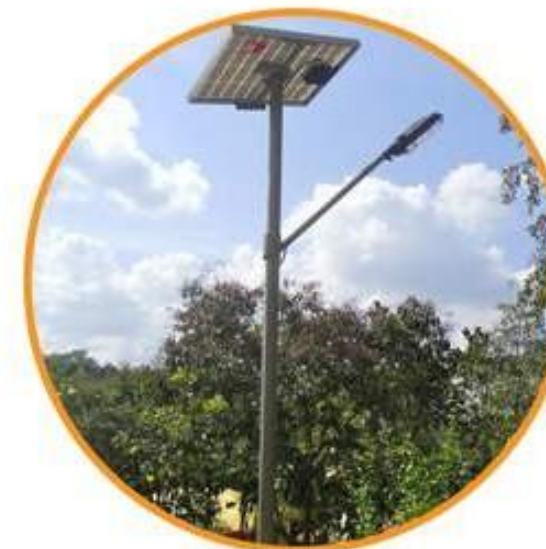
Street Lighting poles and fixtures
